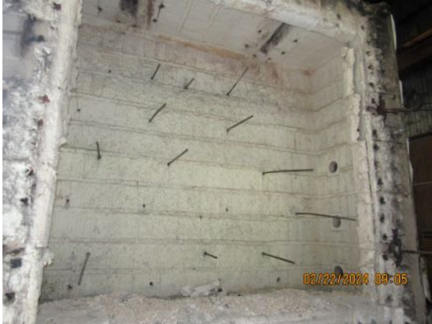
Photo No. 5 View of Burner
