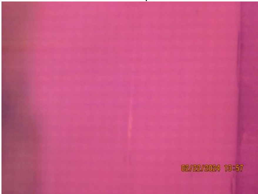
Photo No. 8 Flame in the Seam
