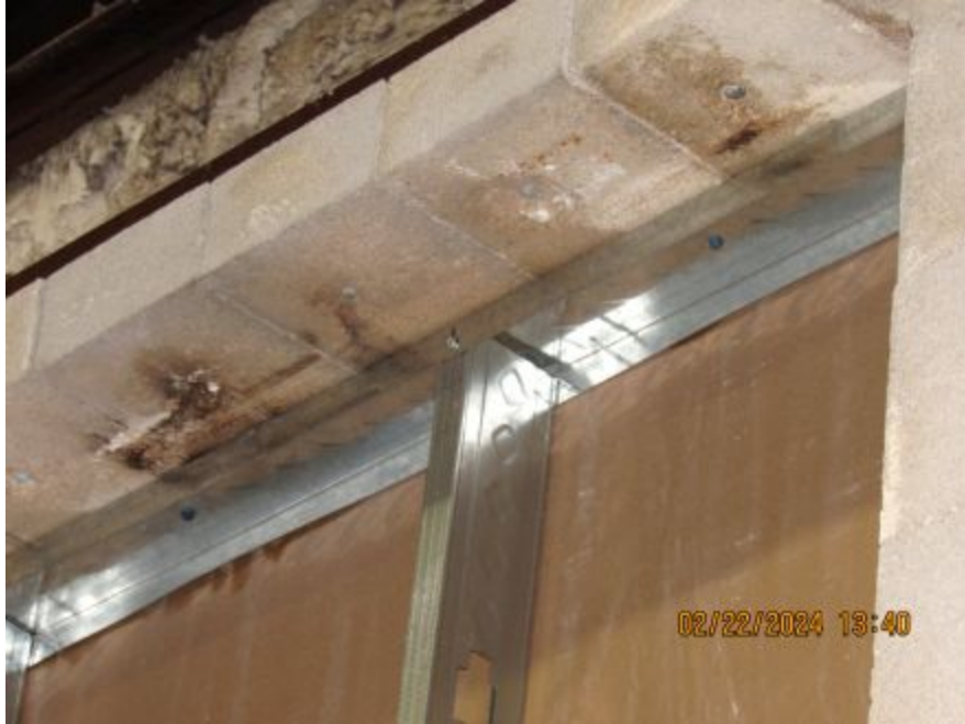
Photo No. 7 Condensation on Top Perimeter
