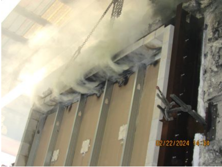
Photo No. 11 Increase in Smoke
